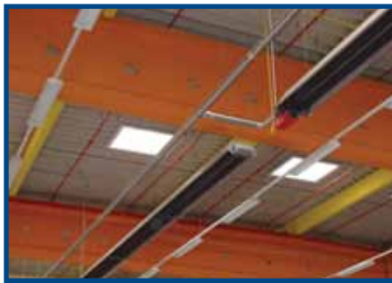
Mechanical and electrical
