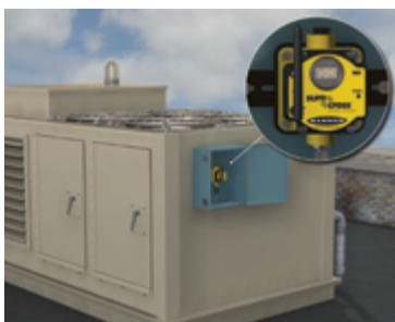
Wireless Control of HVAC System
